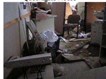
Figure 19: Planning Department offices after Ivan
