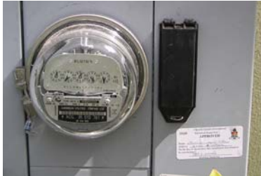
Figure 15: Electrical Meter with a post Ivan approval sticker
