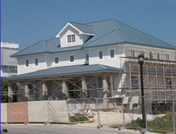
Figure 14: A new home gets finishing touches in the Salt Creek subdivision in West Bay.
