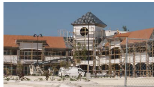
Figure 18: A new mixed-use office and retail center nears completion on West Bay Road.
