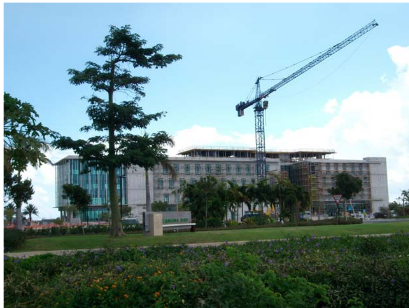
Figure 28: Construction continues at Camana Bay, a “New Urbanist” town off West Bay Road
