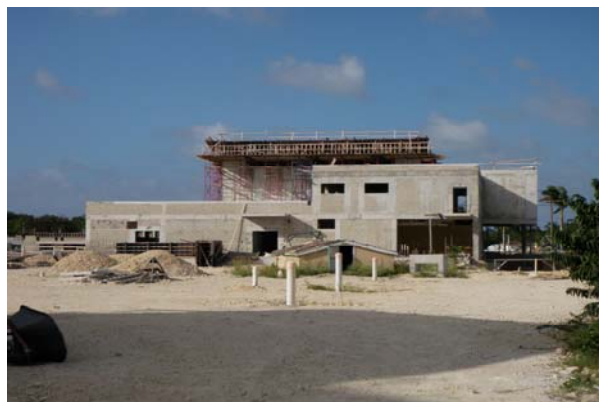
Figure 1 Ia: A new John Gray high school building under construction, off Walkers Road, George Town
