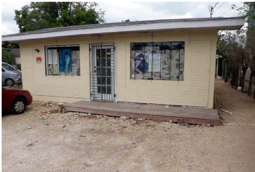
Figure 31: Another compliance matter regarding access to a building.
