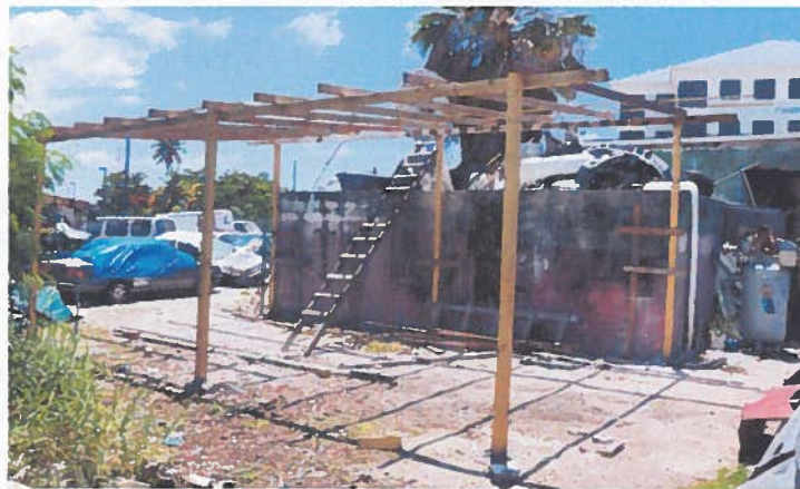
An Example of a Compliance Case (illegal structure)—George Town
