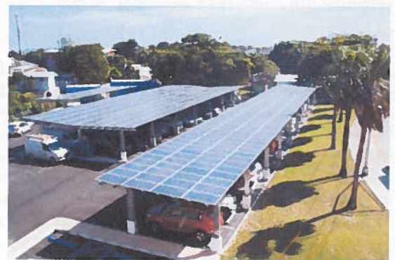
(Ancillary) Solar panel parking shades at Caledonian—George Town
