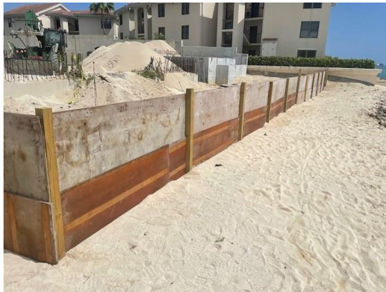
Figure 6: An example of suitable construction fencing to protect turtles (Source: DoE, 2022). Artificial Lighting
