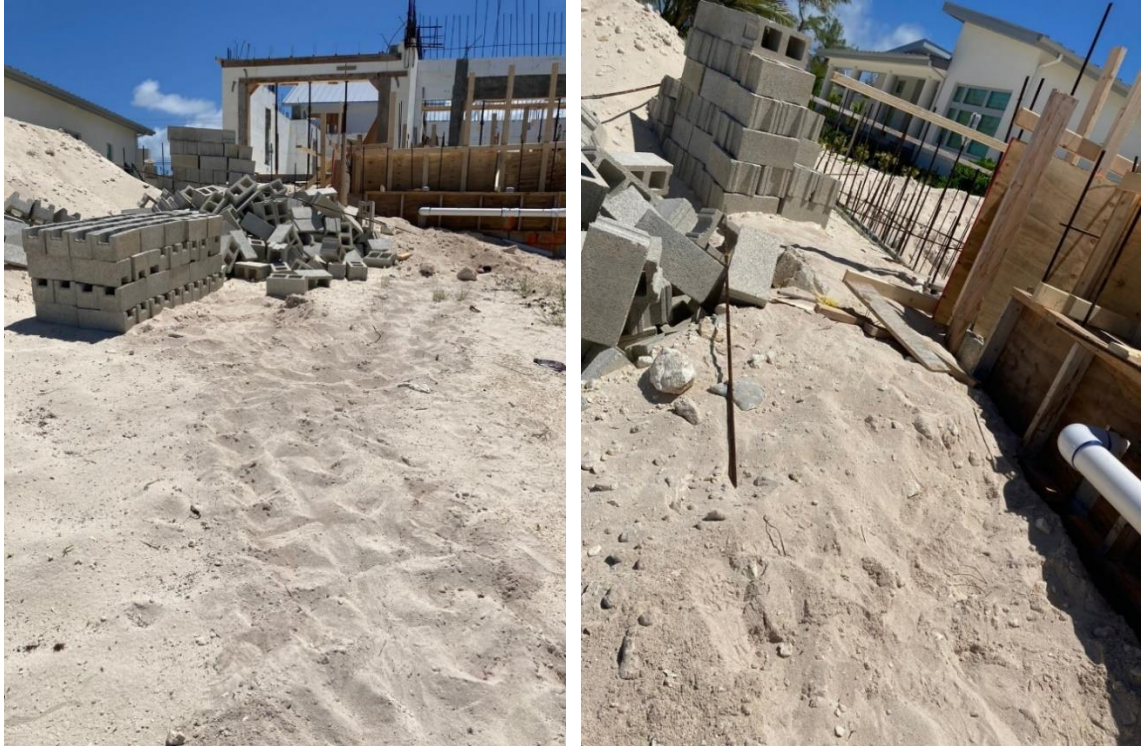
Figures 5-6. DoE photos showing turtle tracks within a construction site on a turtle nesting beach. This site did not have temporary beachside construction fencing to prevent turtles from entering the site. The turtle could have or may have been injured by construction materials and debris on-site (Source: DoE, 2023).
